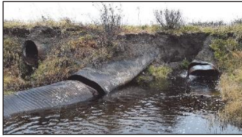
Collapsed culvert under the old, abandoned St. Anthony air strip.
